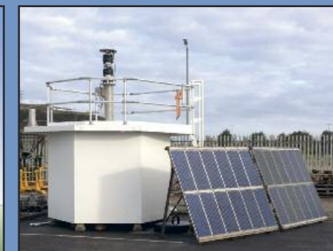
Below: The new aid to navigation on soak test in Swansea Buoy Yard with twin 12 mile light and solar array. The fog signal and radar beacon (racon) are not shown.
