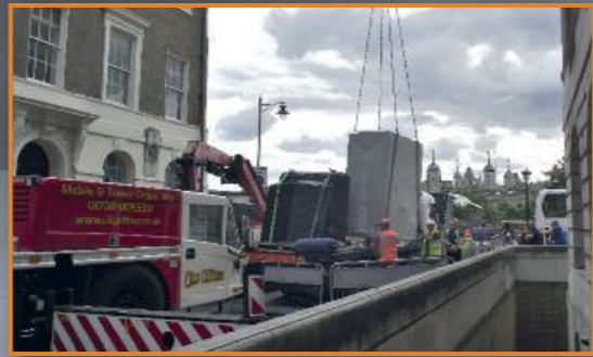
Above: Replacement of the chiller unit which services the air-conditioning to the House being craned in with Trinity Square closed.
