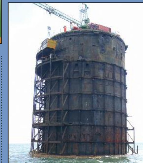
Above: May 2013, the tower crane is erected and extends to the base of the old ammunition shaft. The removal of the old steel framework is progressing.
