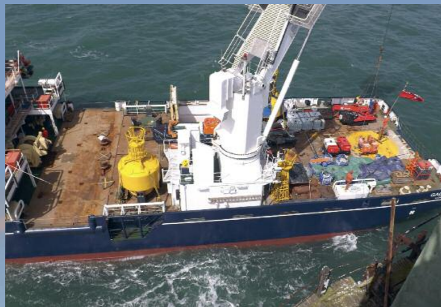
Above: April 2013, THV Galatea loading equipment onto Nab Tower to commence the demolition works. Here the temporary mobile crane is about to be loaded on, the crawler crane was used to erect the tower crane that was central to the works throughout the project.
