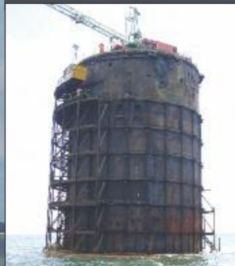
Below: May 2013, the tower crane is erected and extends to the base of the old ammunition shaft. The removal of the old steel framework seen in hand. Photograph ©Ambrose Greenway.
