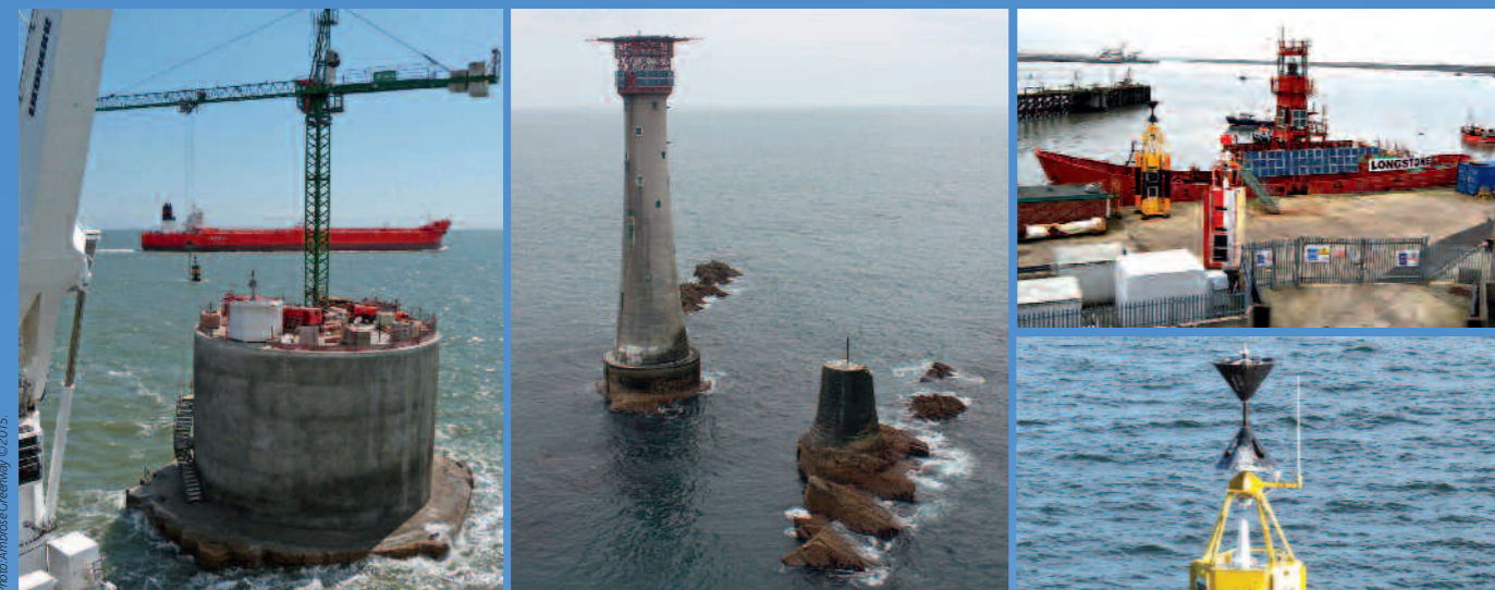
Above and main picture: The principal project of the year was the major civil engineering at Nab as it approached its first century of operation. Works at Nab were the largest capital project in financial terms since the construction of Royal Sovereign lighthouse in 1971 with a budget of £2.5 million.
