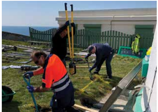
Nick, Rob and Phil hard at work digging foundations for the new solar array
